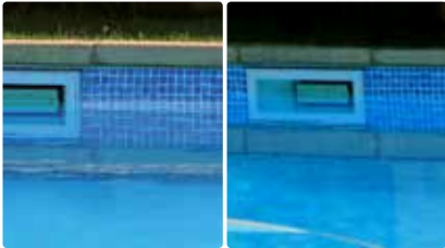
Swimming pool water line
