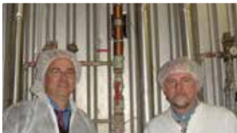
Vulcan installed in a food factory
