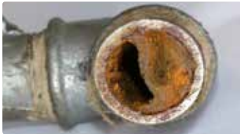
Pipe with scale deposits
