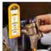
Frame houses labels on Bulk Systems
