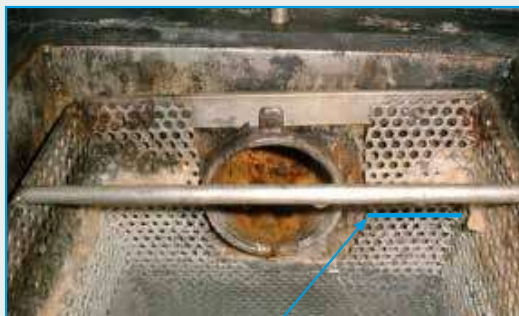
Usual level of standing water.
