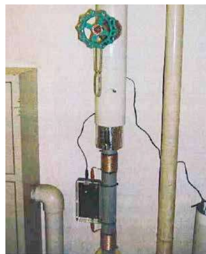
Vulcan 5000 was installed in the factory kitchen
